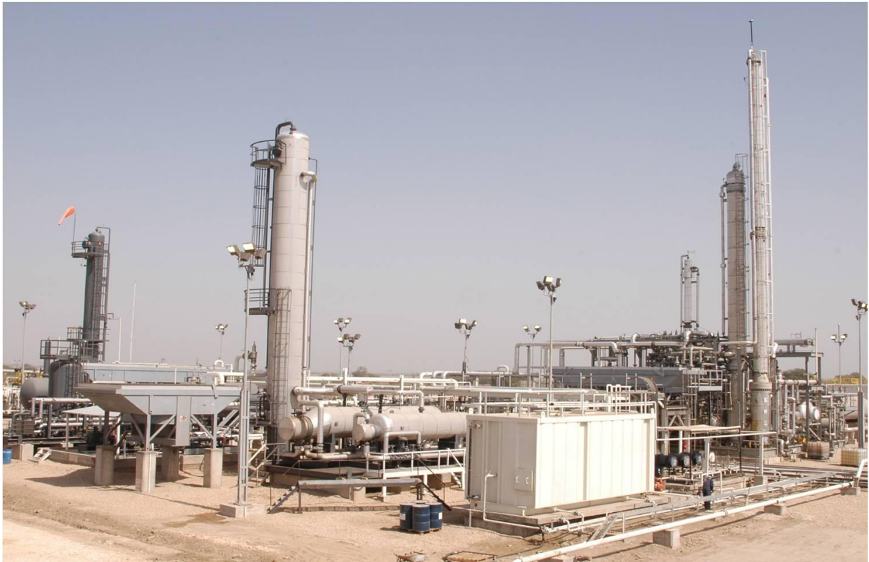
PPL's Hala Early Production Facility
