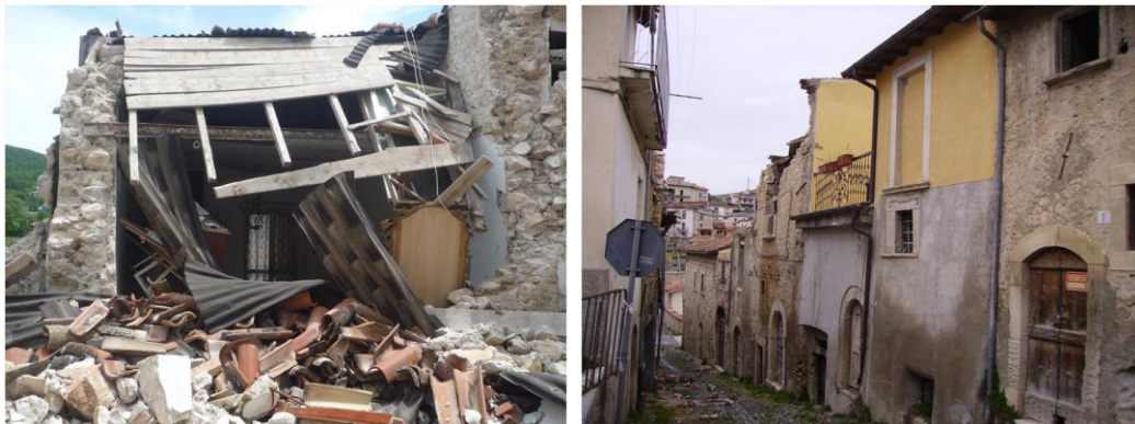
Fig 6. Damages occurred in the historic centre of Poggio Picenze after the 2009 L'Aquila earthquake
