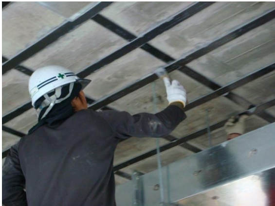
Fig 9. FRP at a slab
